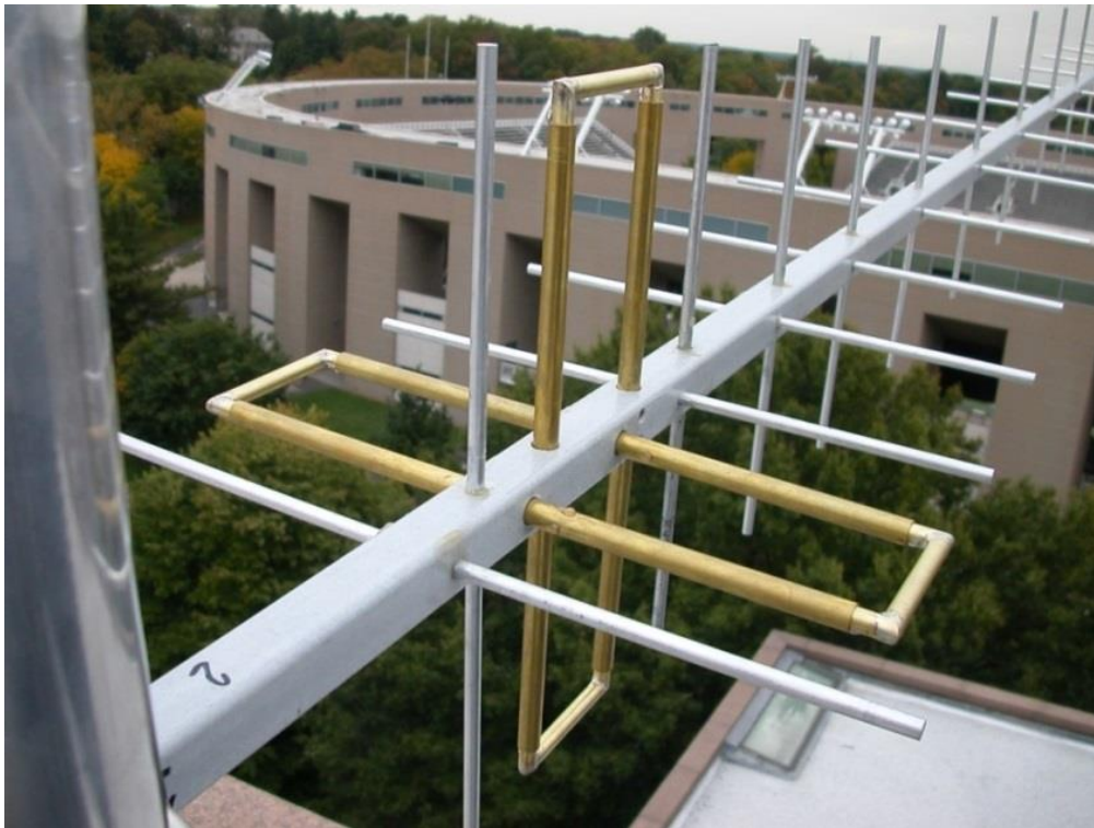
Fig. 4. – Rear view of a single Yagi showing construction details around the driven elements. The brass loops are fed at the split centers of their forward sides, inside the hollow boom. RG142 coaxial feedlines pass out to the rear. All elements are held in place with tight-fitting holes and a few drops of fiberglass resin.
